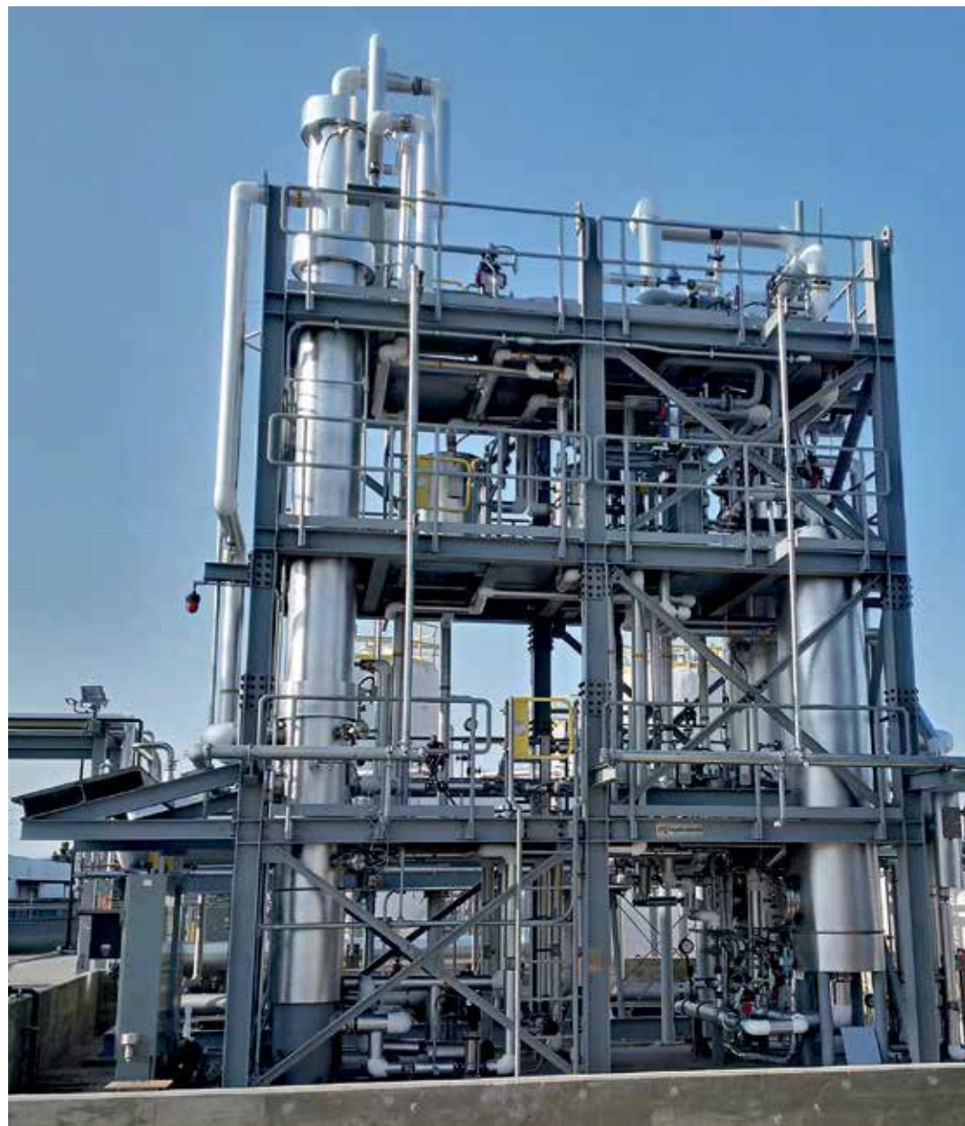
System is installed and ready for operation
